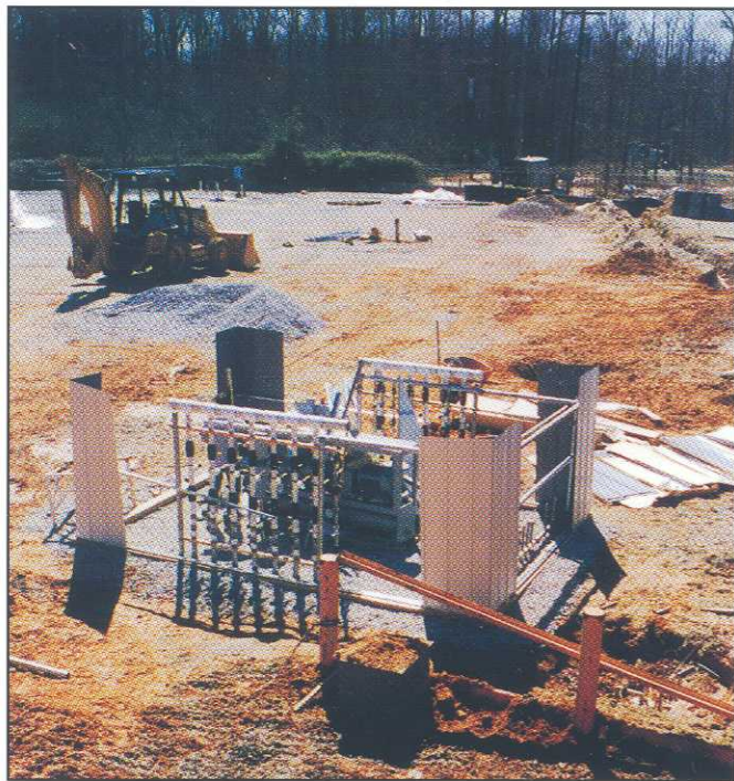
An FE ACTIVE system is installed to remediate DNAPLs at a contaminated site. A combination of technologies applied simultaneously in multiple wells induces strong push-pull forces between wells and through the subsurface formation zones targeted for remediation.
